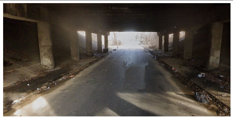
Brown Ave. underpass in Klondike: Inadequate sidewalk and no bike lane
