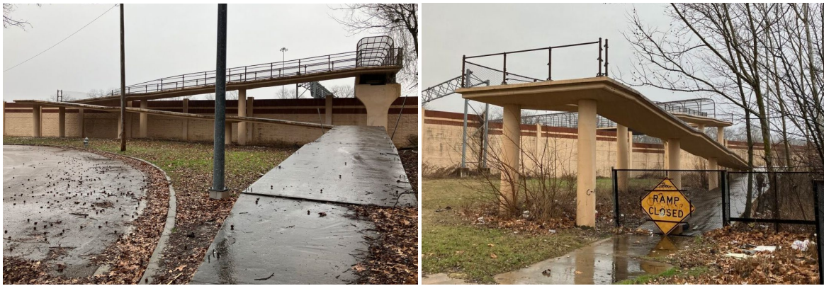
Hazardous pedestrian overpasses in Smokey City (left) and Klondike (right) missing large sections of railing.
