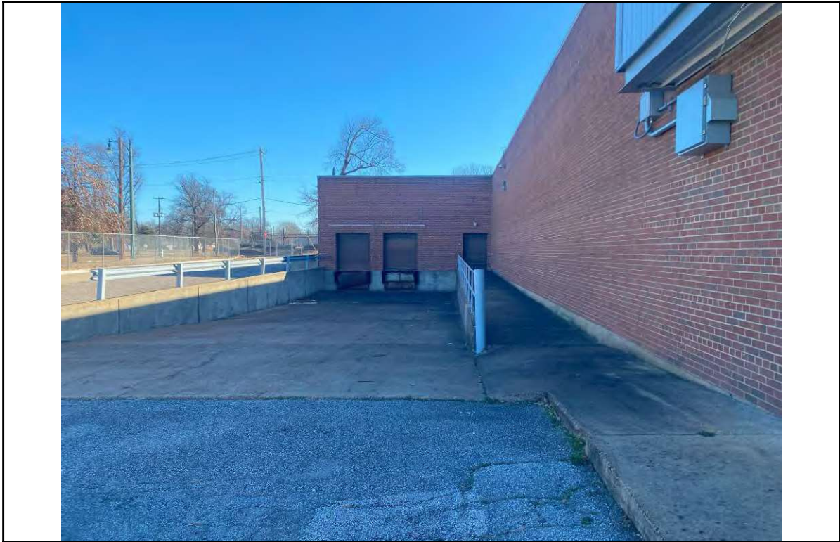
PHOTO NO. 6 DESCRIPTION: View of the recessed loading dock on the north side of the subject property building.
