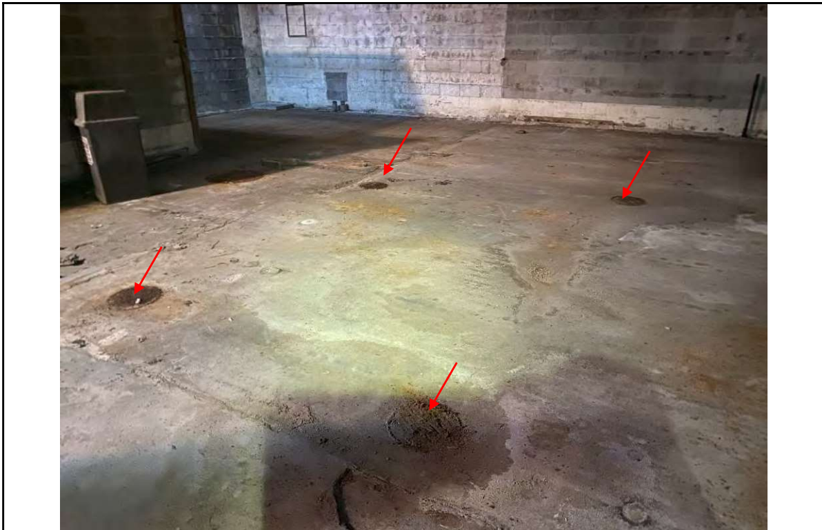
PHOTO NO. 4 View of some of the floor drains (arrows) observed within the subject property building near the former restroom area. Also, note the rust and white colored staining on the concrete floor. DESCRIPTION:
