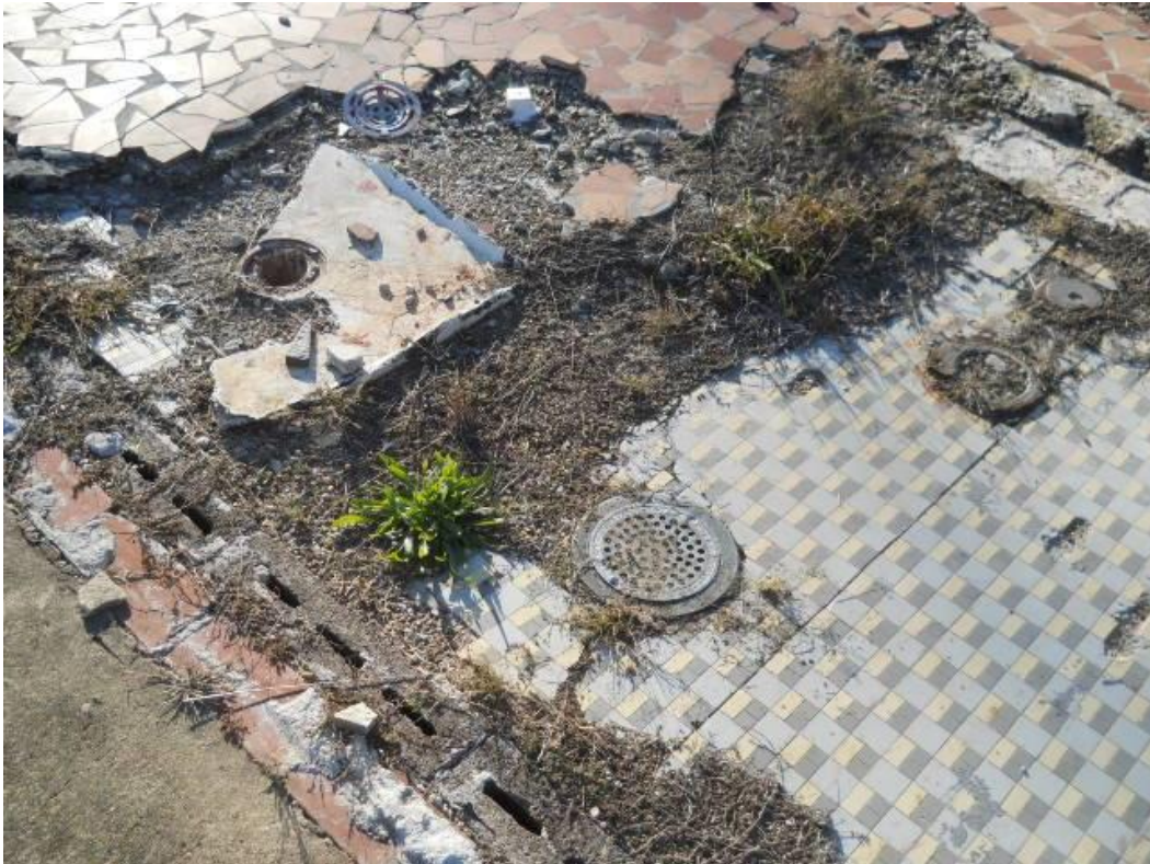
Photo #39 View of two of four interior floor drains located on the former Wayne's Pinball Palace concrete slab foundation
