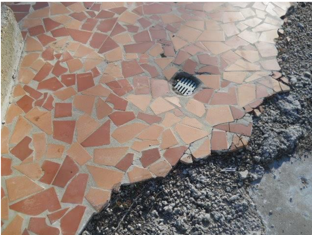
Photo #38 View of one of four interior floor drains located on the former Wayne's Pinball Palace concrete slab foundation
