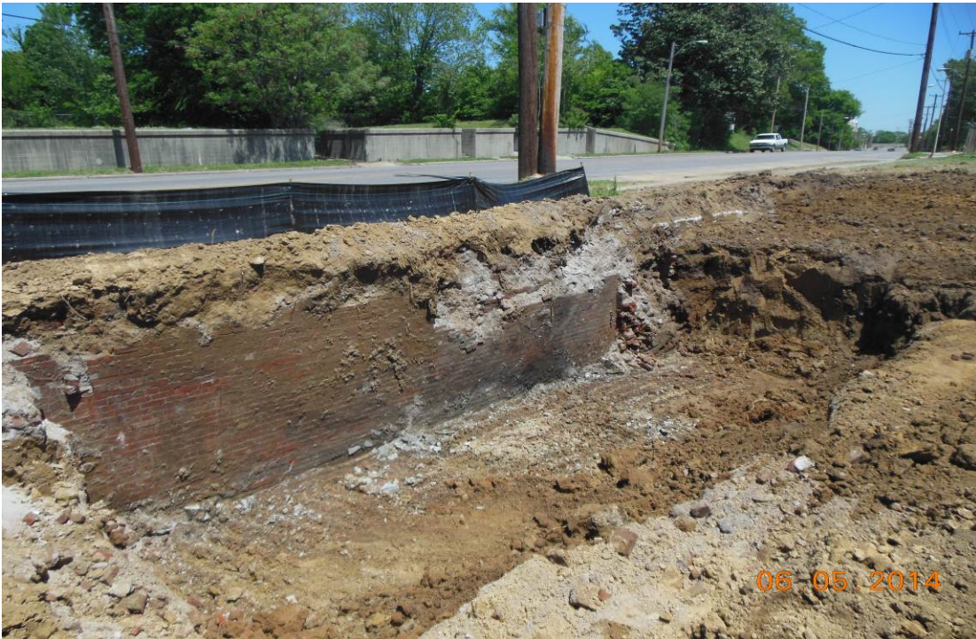
Photo 10: Final debris removal from Basement #2. Brick foundation wall pictured remains onsite, to ensure right-of-way is not damaged.
