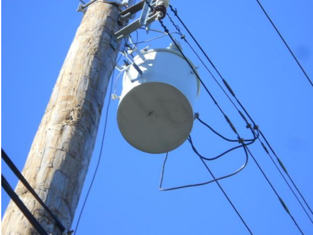
Photo #51 View of the pole-mounted transformer located southwestern most corner of the site
