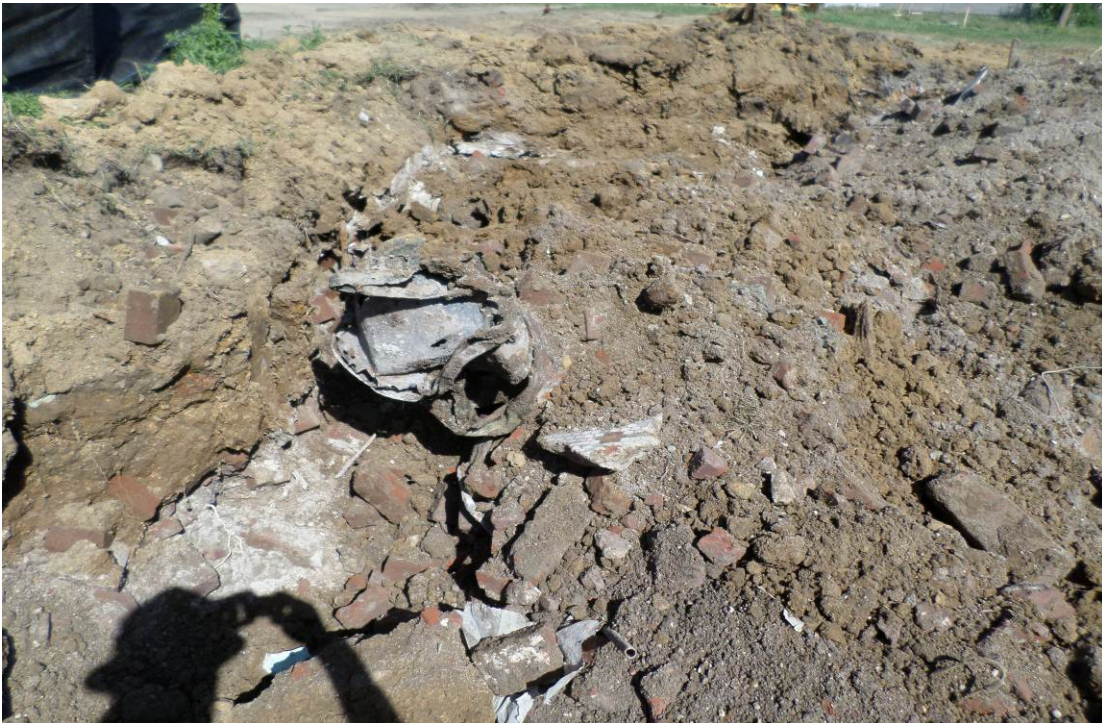
Photo 6: Removal of debris from Basement #2. Hot water tank is pictured here.
