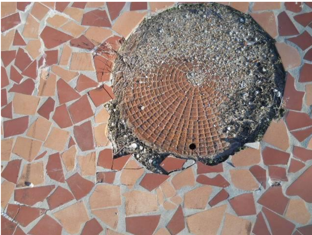
Photo #40 View of the manhole located inside the former Wayne's Pinball Palace building foundation
