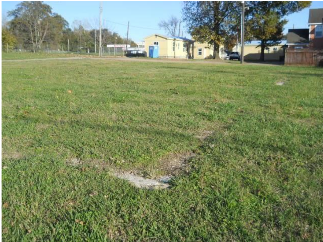
Photo #46 View of a concrete footer associated with a former structure located in the southeast block of the site
