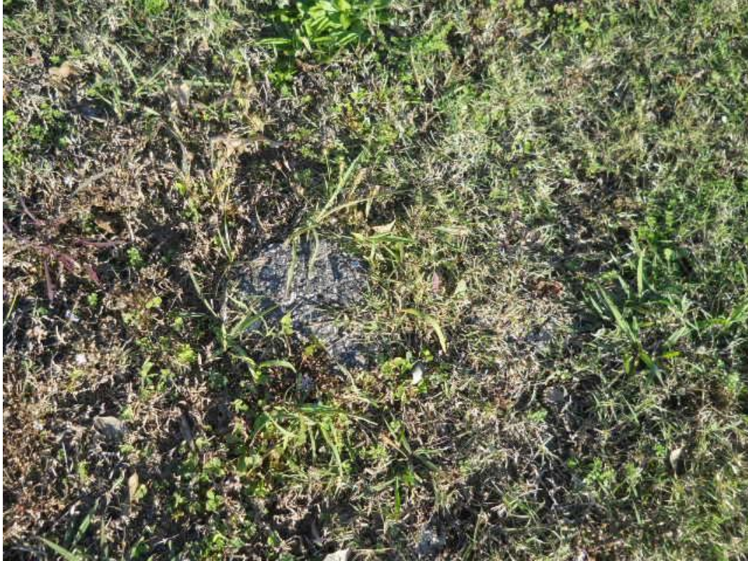
Photo #49 View of asphalt debris located in the northeast block of the site
