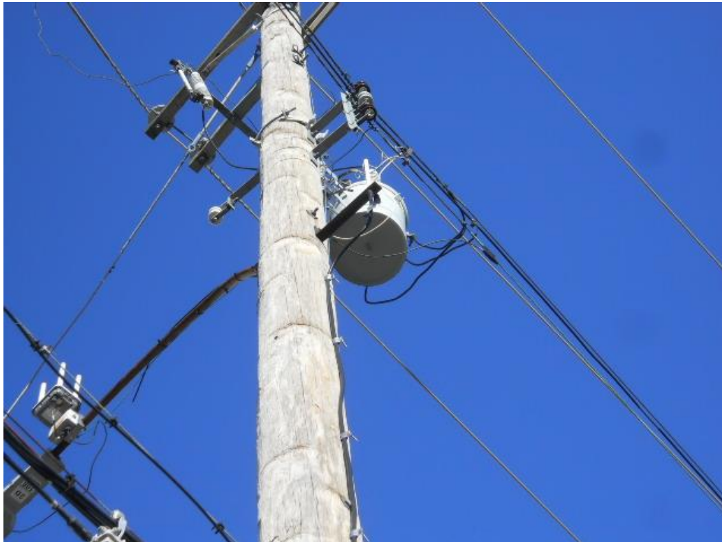
Photo #50 View of the pole-mounted transformer located along the northern boundary of the site
