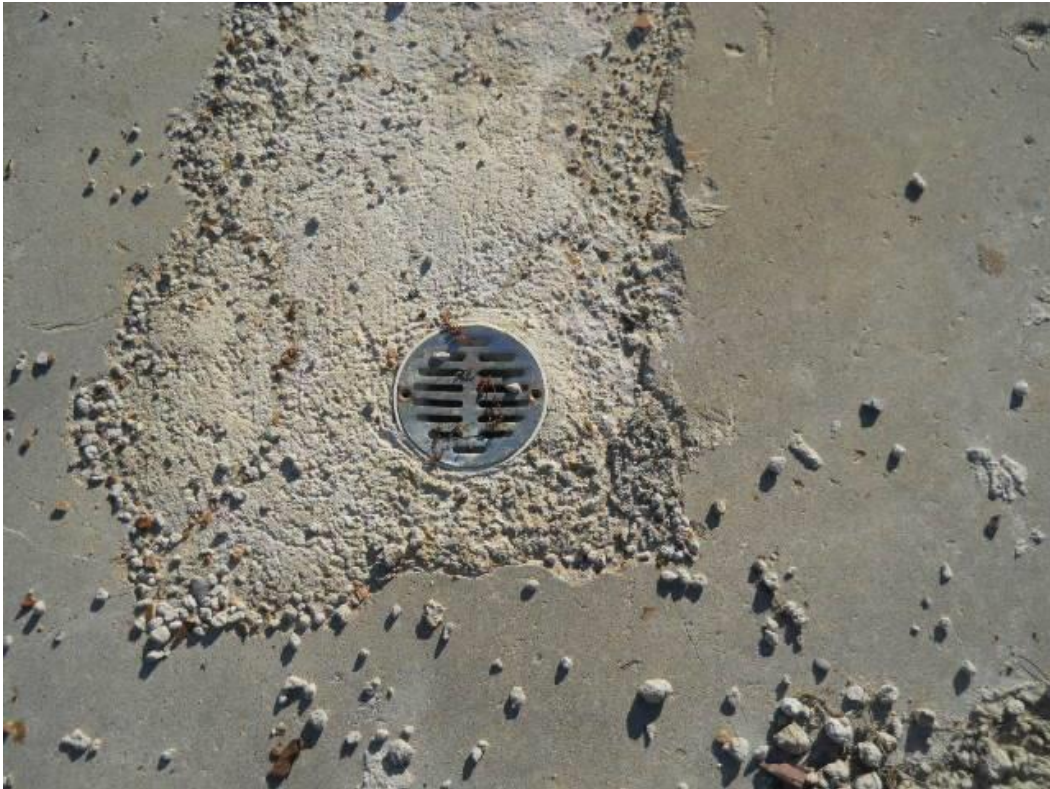
Photo #37 View of one of four interior floor drains located on the former Wayne's Pinball Palace concrete slab foundation
