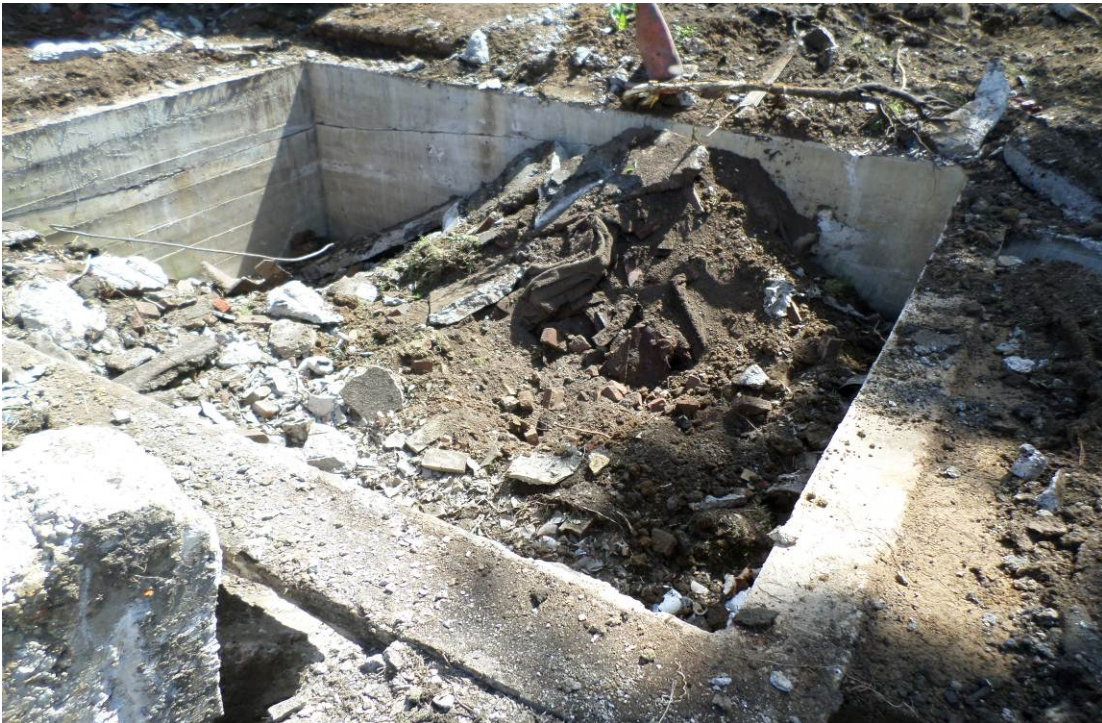
Photo 4: View of all delirious materials still inside Basement #1.
