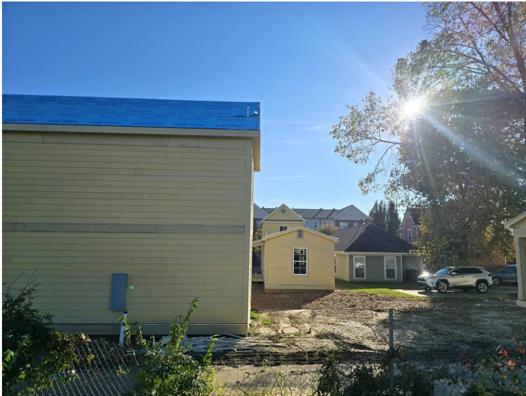
Photo #34 View from the site of looking south towards the residences which area under construction south of the northeast block of the site
